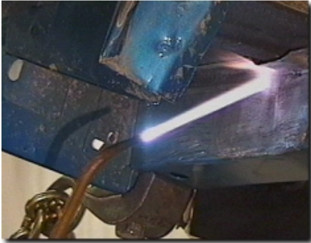
B-5 Applying heat can reduce the strength of metal temporarily while straightening methods are applied.
